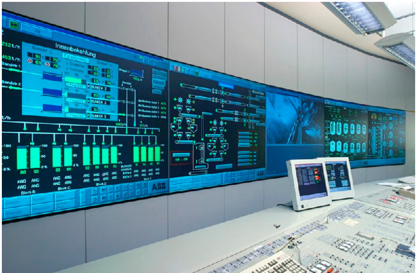
Figure 1. Controller System Room
