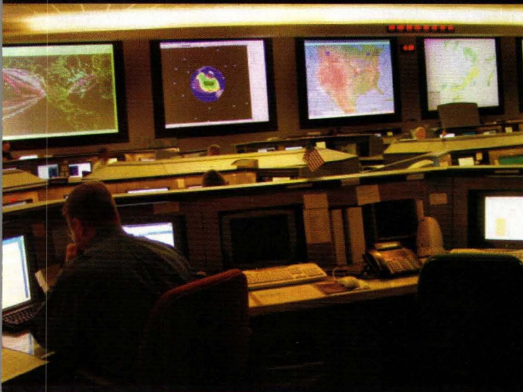
Herndon Control Center, Virginia
