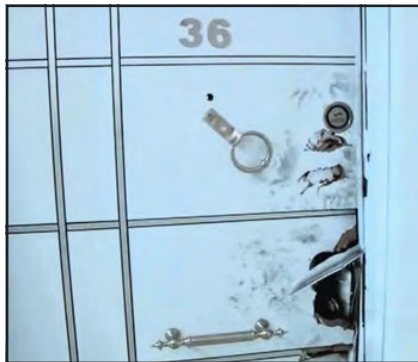
Damage is evident on the front door of the safe house after police had gained entry
